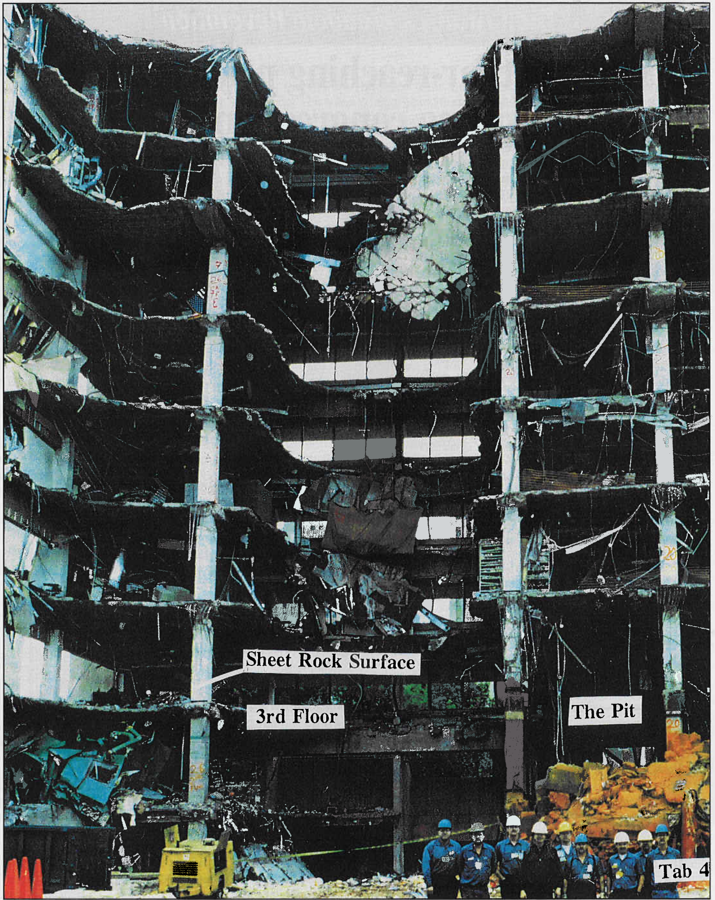
The partially cleaned up structure in "Tab 4" of Partin report shows that the failure line across the roof goes all the way to the ground except around columns B4 and B5, where large areas of the 2nd and 3rd floors (labeled "The Pit" here and in "Tab 2" diagram) were taken out by the truck blast. Most of the sheetrock on column B4 is still intact, although B3 failed.
