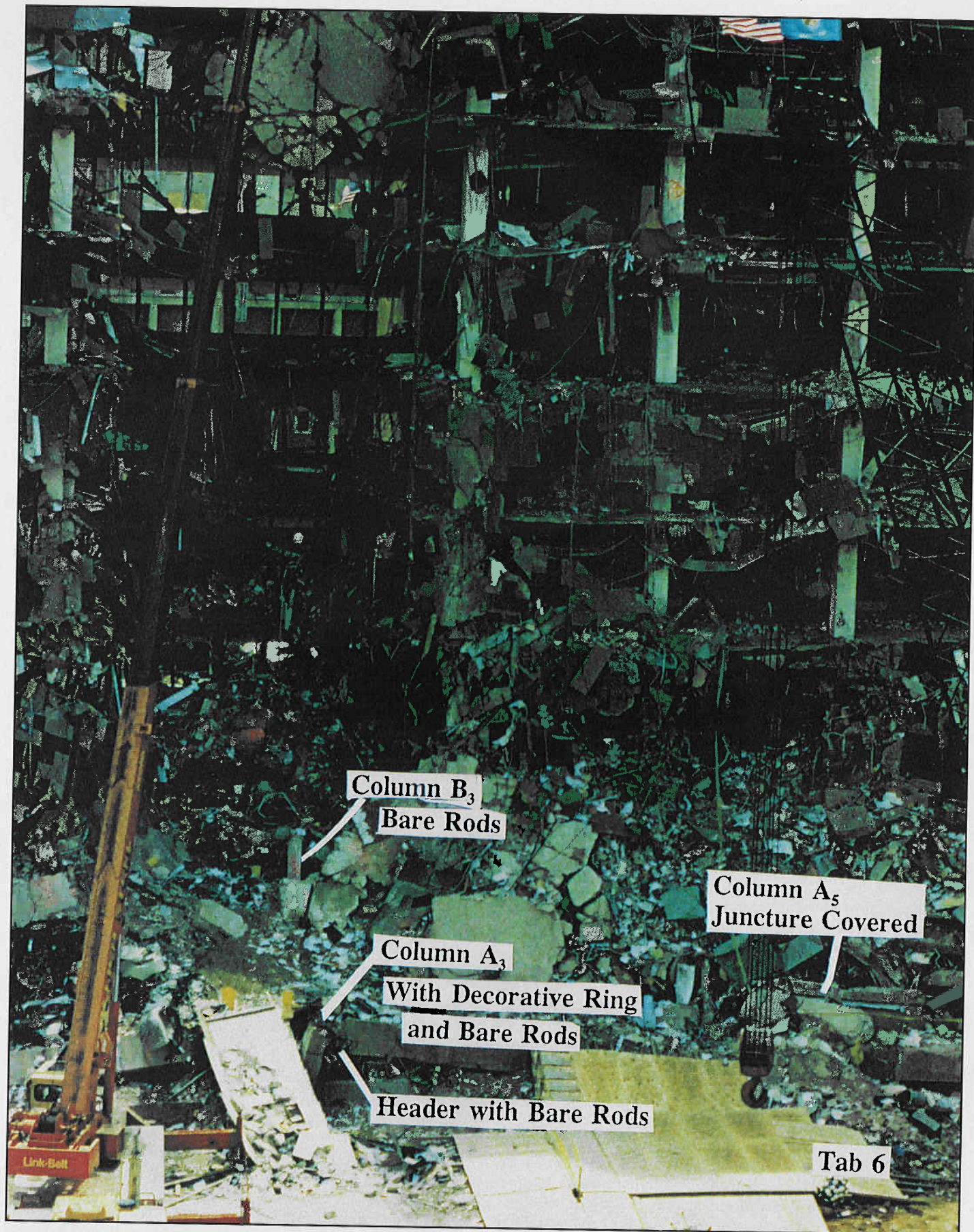
The stub of column B3, which was completely removed in "Tab 4," is visible here in "Tab 6." Close examination shows bare re-bar at top of stub, corresponding to 3rd floor level. Smooth failure and bare re-bar also visible at header end to the right of column A3 indicates demolition charge damage.
